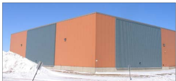
Blue-grey solar cladding installed on the south-east and southwest walls of Building 60.
