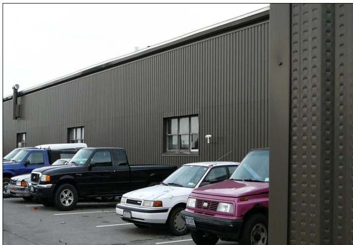
Brown SolarWall panels on the south façade of Building 91.
