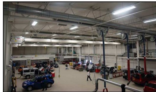
Inside the Jaguar / Land Rover Academy; SolarWall ducts distribute the solar heated air throughout the building.
