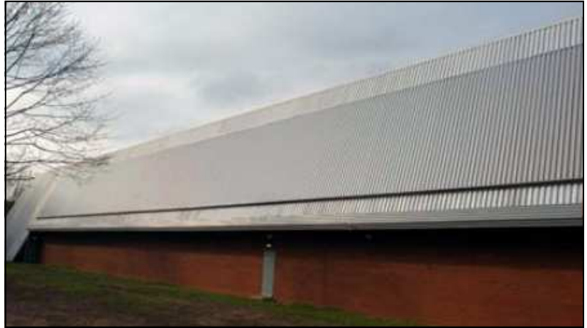
The grey SolarWall® solar air heating system integrated into the southern façade.
