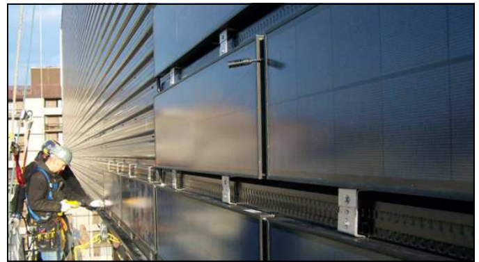
A close up of the SolarWall® PV/T system's custom Day4 photovoltaic modules being installed over the black metal SolarWall® system.
